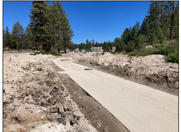
More construction at Snow Valley near Deep Creek, a federally designated wild and scenic River.
