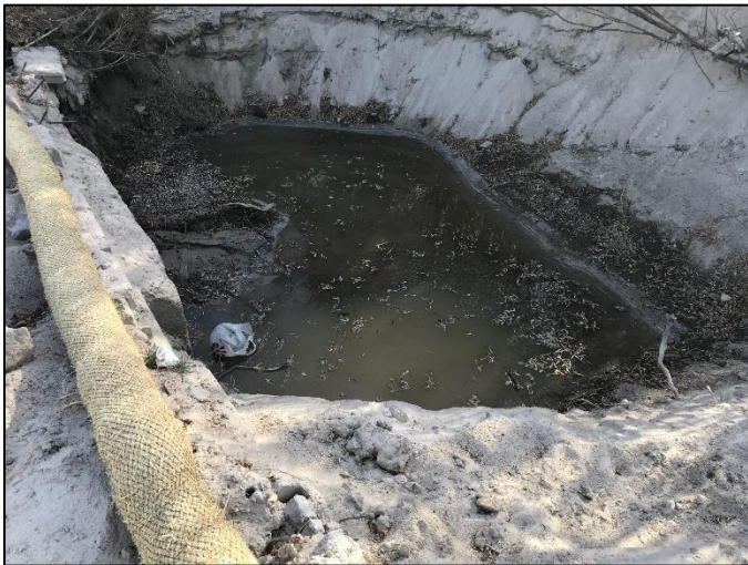
Current construction in Snow Valley Parking lot indicating ground water contamination.
